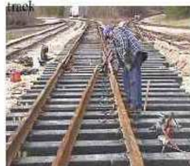
Plastic composite ties in turnout
